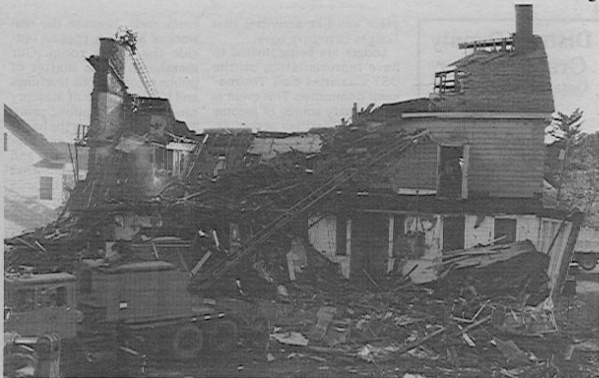
Heavy construction equipment was brought in to assist firefighters. The building was considered too severely damaged to allow the walls to remain standing.
