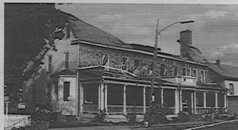
The front of the building following the fire, with the severely damaged roof partially collapsed.
